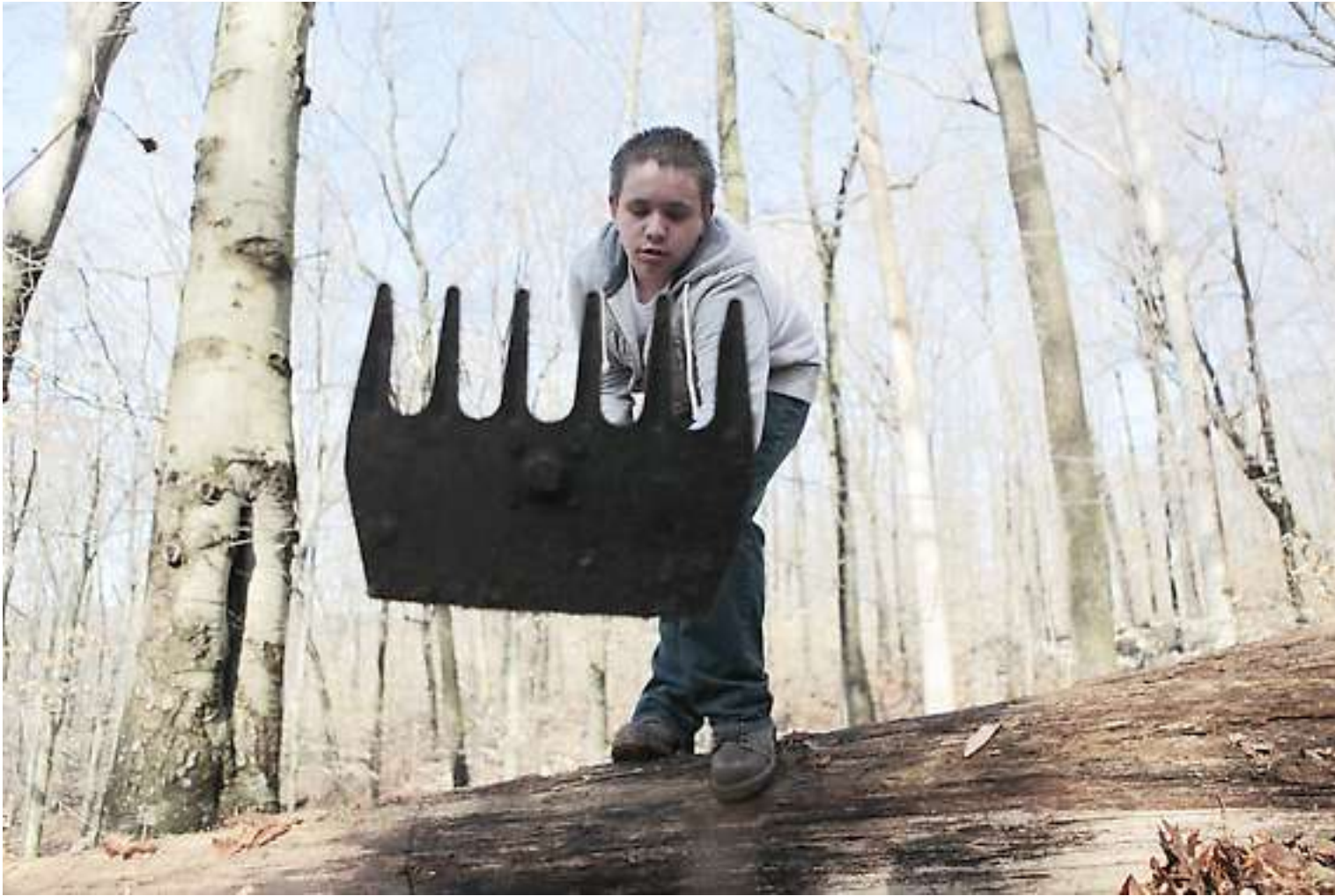
Cassey Lene helps build a trail near Lake Lemon. TOP: A Cranefly orchid is relocated from a trail to a different place in the woods owned by Sycamore Land Trust that's north of Lake Lemon. Jeremy Hogan | Herald-Times
